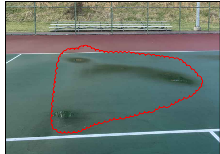
#6 Repair low spots- ponding water. Patch w/ Latex-Ite Acrylic Patching & Leveling Compound
