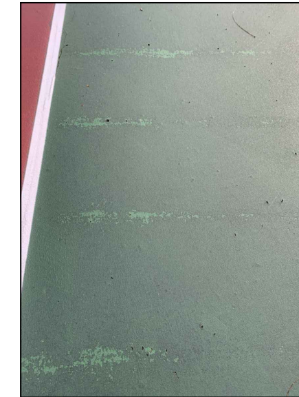
Typical- wear in surface Repair as required to prep for resurfacing.
