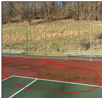
#4 Repair low spots- ponding water. Patch w/ Latex-Ite Acrylic Patching & Leveling Compound
