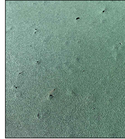
#11 Typical- repair pitting throughout as required for resurfacing prep
