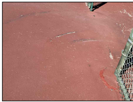
#1 Scratches from gate & crack repair typical around posts
