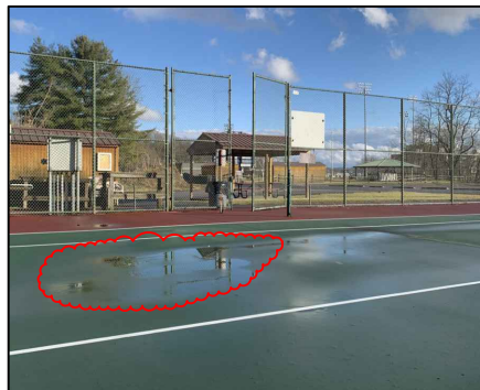
#2 Repair low spots- ponding water. Patch w/ Latex-Ite Acrylic Patching & Leveling Compound
