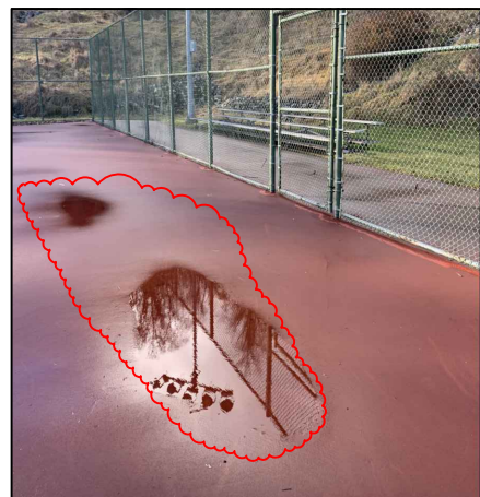
#7 Repair low spots- ponding water. Patch w/ Latex-Ite Acrylic Patching & Leveling Compound
