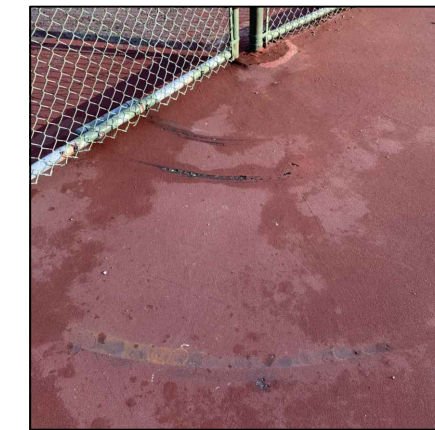
#13 Scratches from gate & crack repair typical around posts
