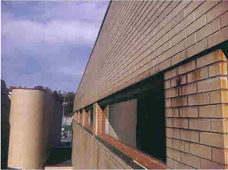
Fig. 3 Brick façade movement at clearstory
