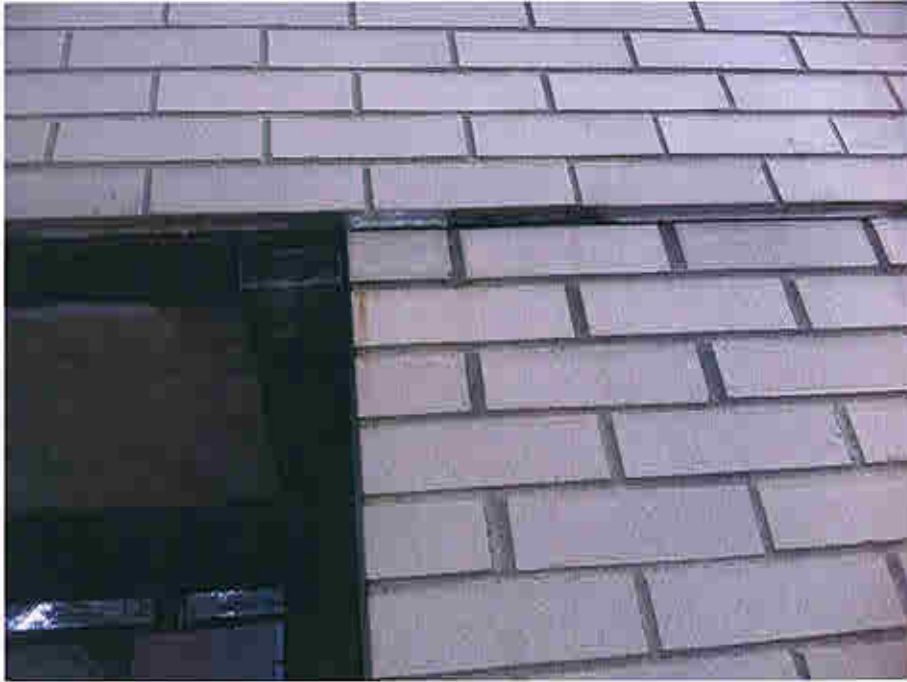
Fig. 5 Brick movement at sliding glass doors
