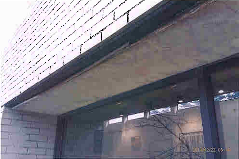
Fig. 7 damage at lathe and plaster soffit
