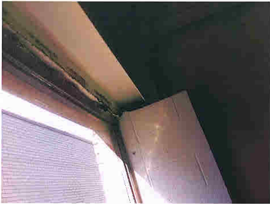
Fig. 1 showing red iron corrosion at clearstory
