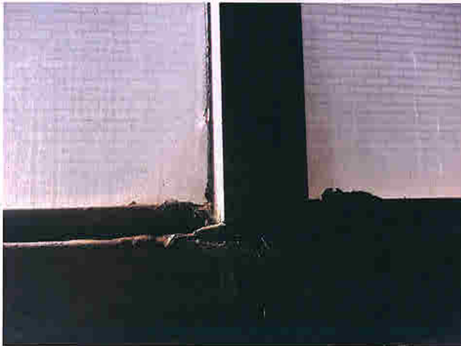
Fig. 2 showing corrosion at clearstory window frame
