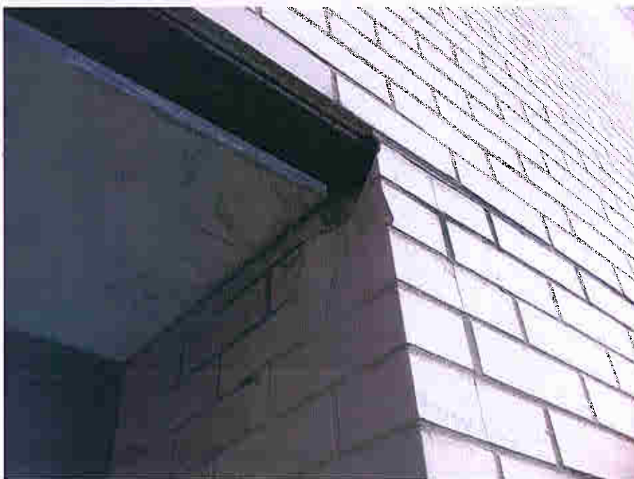
Fig. 6 Cracked and broken brick
